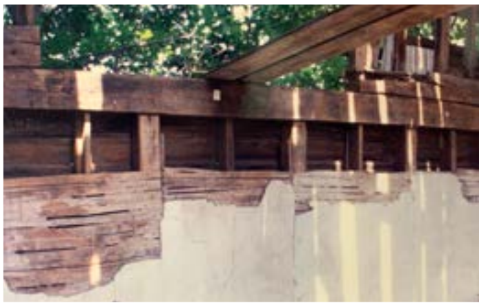
Wall of former Methodist Church, circa 1818 in Wellandport. The hand split lath (narrow horizontal wood pieces) holds the remaining plaster on the interior, with clapboard on the exterior walls. Note the hand split lath with remaining plaster inside & clapboard outside (without board sheathing).
