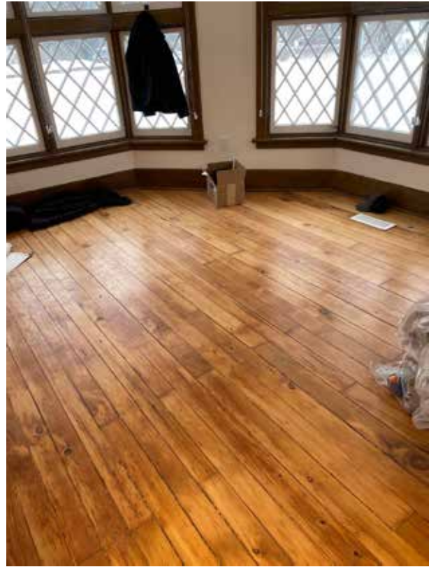
Restored floor in the stable hands quarters with original "wavy" or antique glass windows
