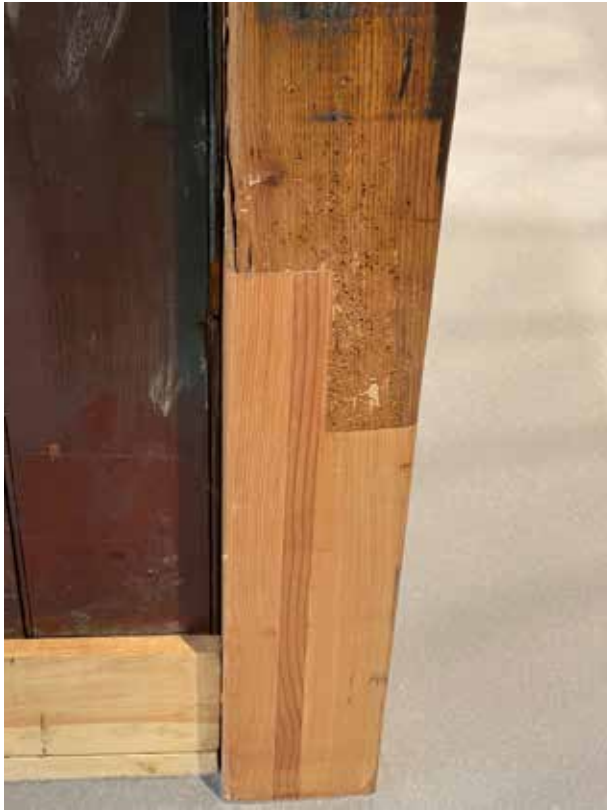
Damaged wood is replaced with salvaged wood of similar age, same species
